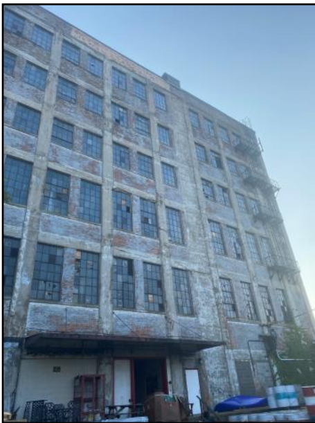
The old Hunt's flour mill behind Nova Craft Canoe, August 26, 2021. The short, stubby chimney is on the edge of the roof. (photo by Brendon Samuels)
