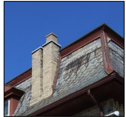
Close up of chimney used by swifts at 423 Colborne. Swifts entered the shaft through the "pot" on top of the chimney shaft on the right.
